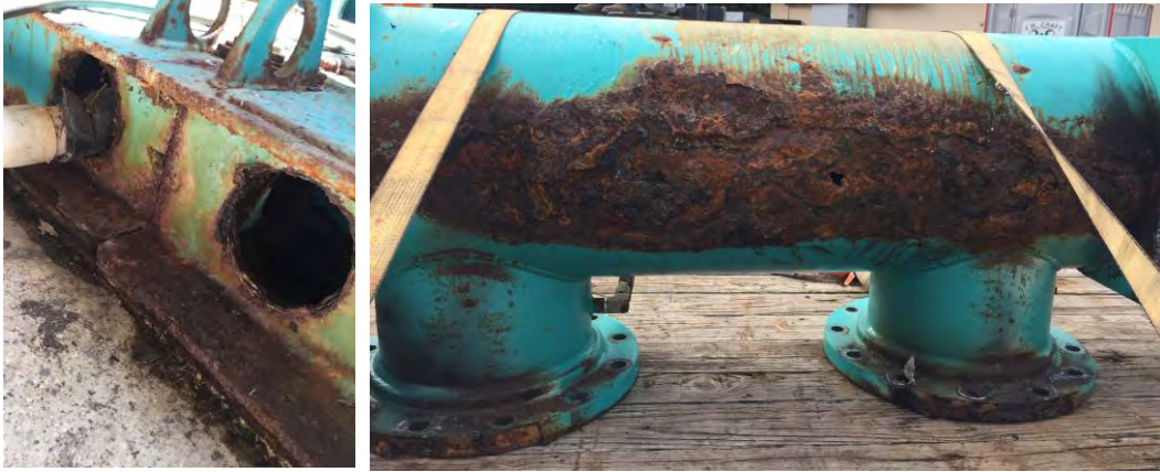
Examples of corrosion in the old station.
