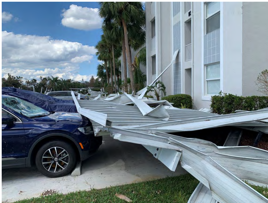
Carport damages outside Terrace building #10 on Butterfly Palm Drive.
