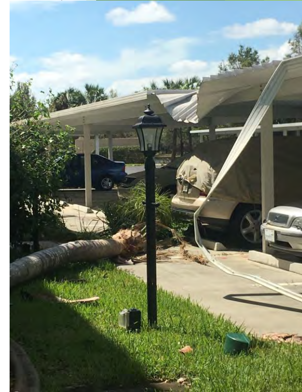
Car port damage.
