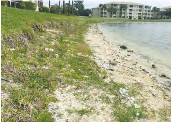
Shoreline erosion along the west side of Lake 8 (the Big Lake) was accelerated by Hurricane Irma.
